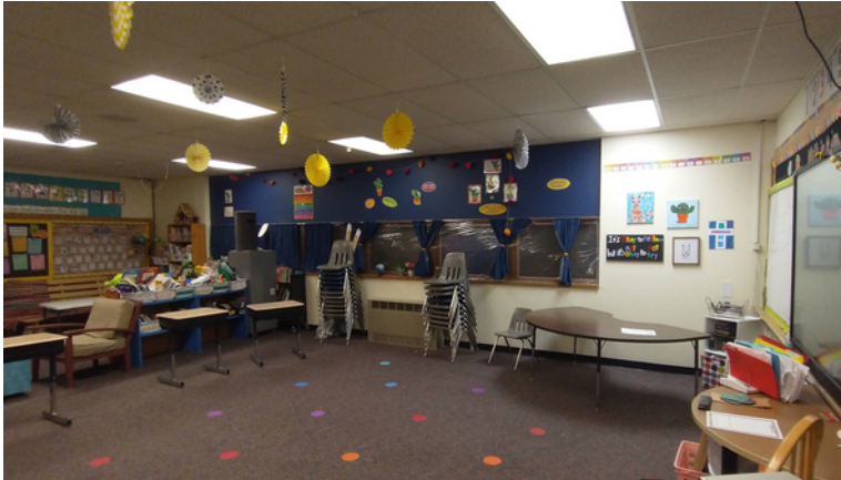
Before: Small windows, low ceilings with outdated lighting, plastic on windows to conserve heat.
